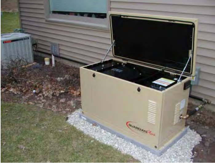
Fig. 14.2. A 7-kilowatt standby generator installed outside of a house, next to the air-conditioner. A 20-kilowatt cold fusion generator will be roughly this size. Photo by D. Kontac in product review on Amazon.com.
