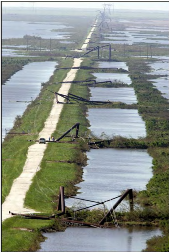
Fig. 14.1. Power lines damaged by a storm, Florida 2004. Power distribution lines are the Achilles heel of the power companies.
